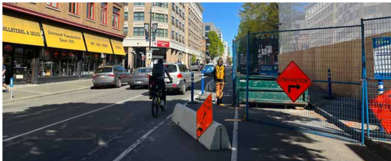
Temporary, protected pedestrian walkway with cyclist taking the lane (permitted for painted bike lanes only).
