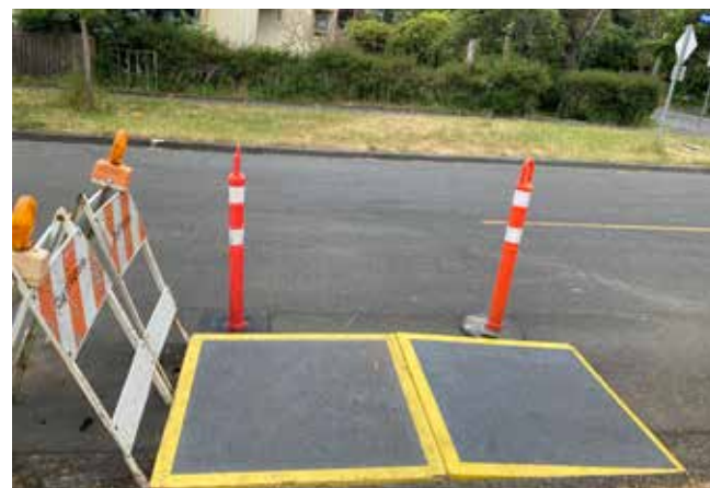
High contrast, non-slip temporary curb ramp provides access to the sidewalk for mobility devices users
