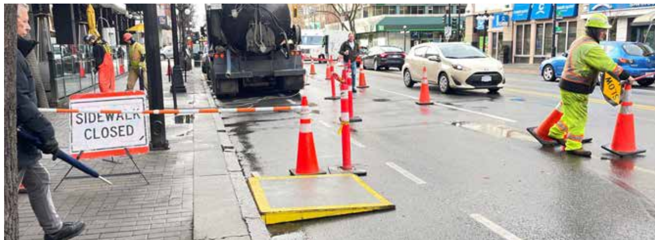
High contrast, non-slip temporary curb ramp provides access to the sidewalk and a temporary protected walkway for mobility devices users
