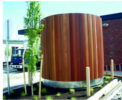
Cistern that fits into a commercial area
